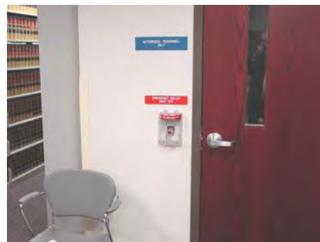
Fire Alarm in Law Library
